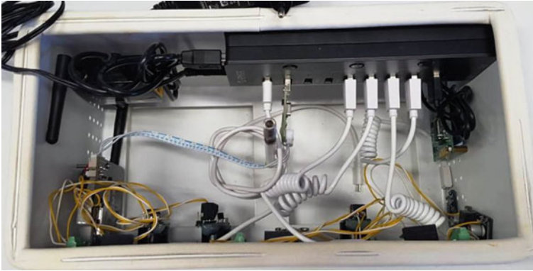
Fig. 11 Sensors, smart router and connectors
